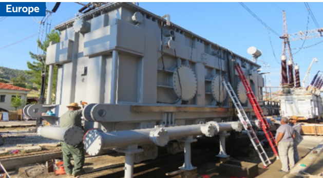
Greece | Greek Power Transmission Company 400kV 280MVA Autotransformer Project
