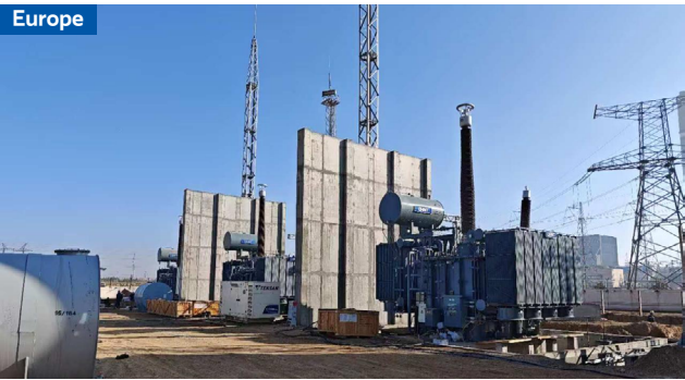
Uzbekistan | 500kV 167MVA Auto Transformer for TIES 1700 MW Talimarjan TPP
