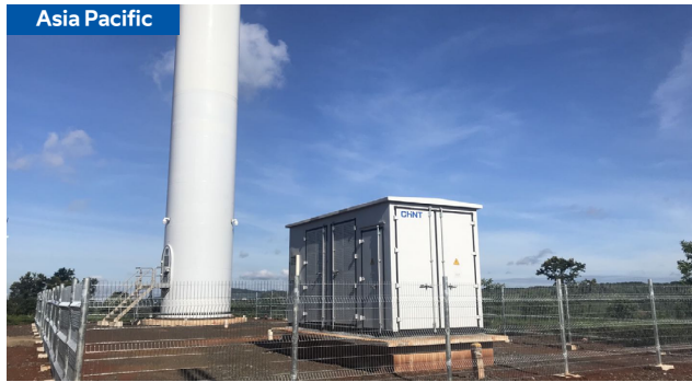
Vietnam | Gia Lai 100MW wind power project
