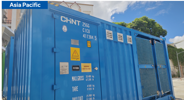
Philippines | Manila Data Center Project
