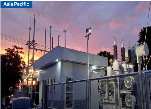
Philippines | ORMECO 10MVA 69kV Naujan Substation
