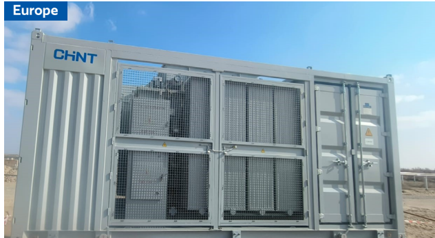
UK | Nur-Bukhara PV Solar Project with Battery Energy Storage System (BESS)
