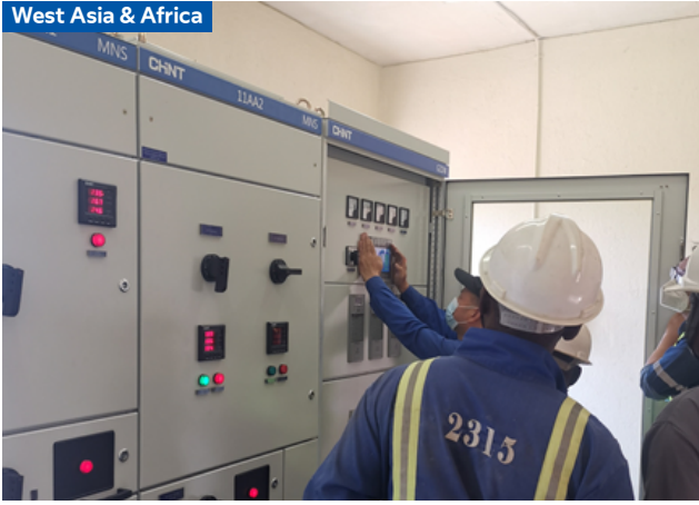
Malawi | DCA International Airport Distribution Grid Upgrade EPC Project
