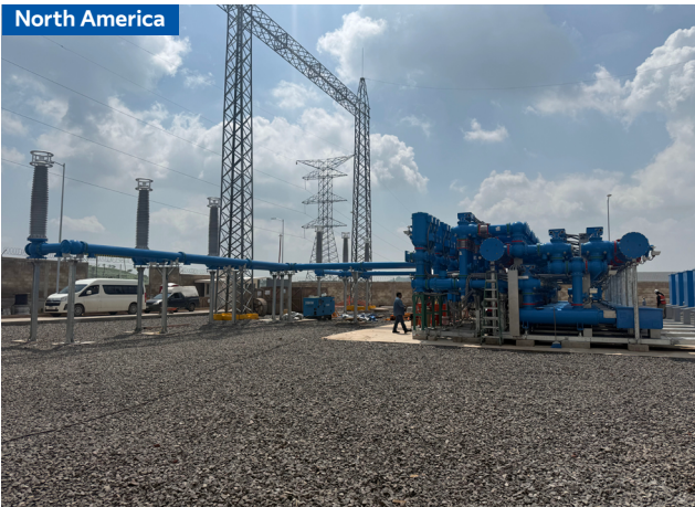
Mexico | PLATAFORMA PARK Project 245kV GIS
