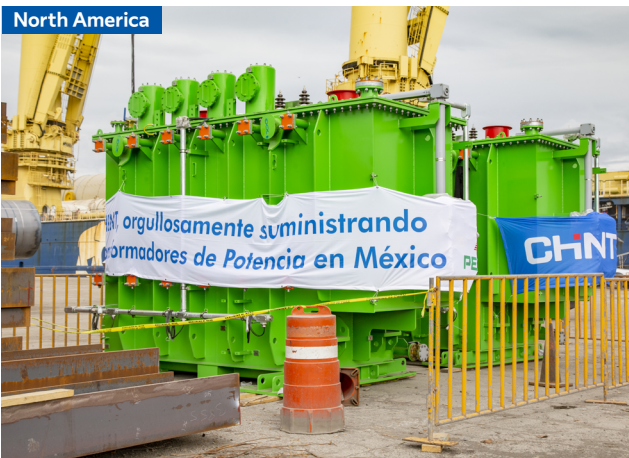
Mexico | PEMEX 115kV Power Transformer Project
