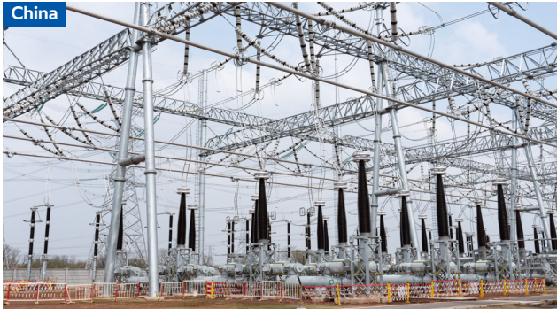
China | State Grid Hengyang 500kV Substation Project
