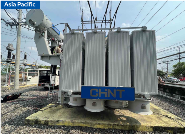
Philippines | PELCO II 69kV Mabiga Substation
