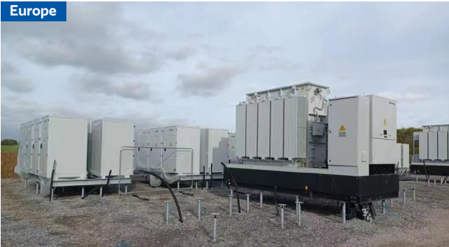
UK | 11-33kV Skids for Trina BESS project
