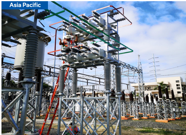
Philippines | NGCP Compostela (CEBU) Substation
