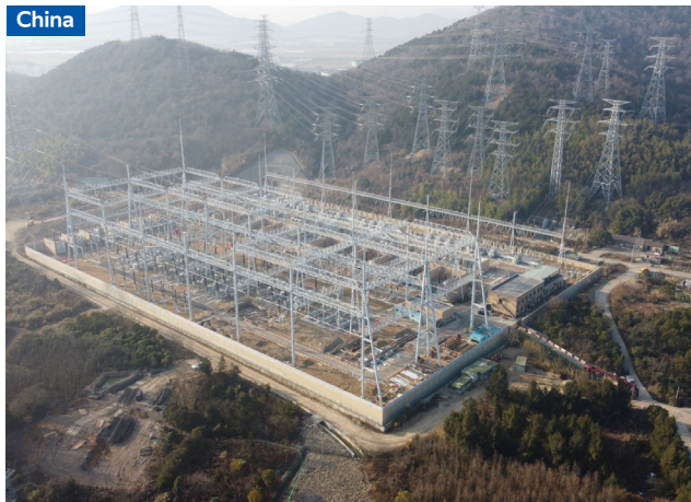
China | State Grid Zhoushan Luojia 500kV Substation Project
