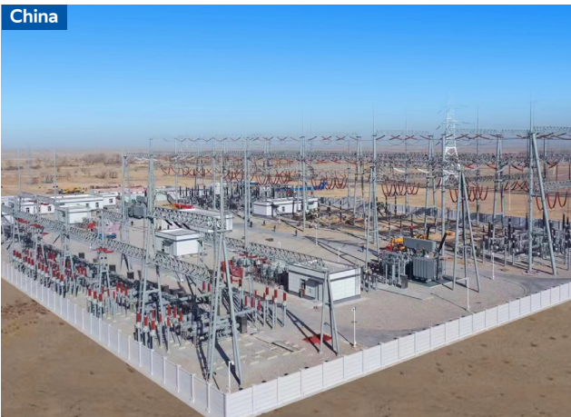
China | State Grid Jiuquan Huahai 330kV Substation Project
