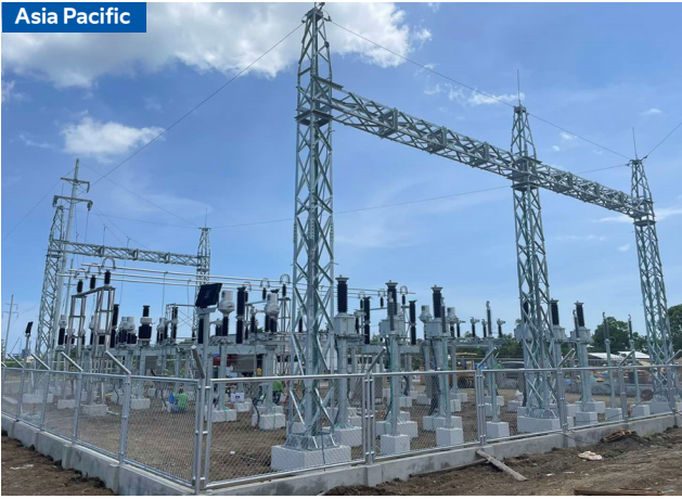
Philippines | DMCI 69kV Narra Palawan Switchyard Project
