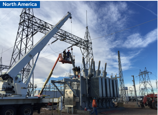
USA | WAPA Archer Substation 230kV 200MVA Autotransformer Project
