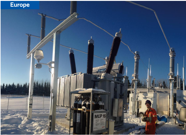
Serbia | 400kV Variable Shunt Reactor (VSR) Project
