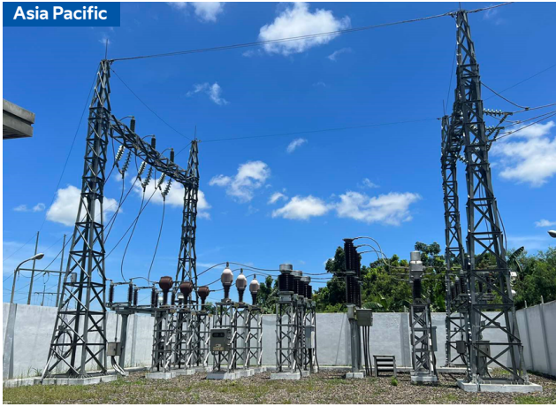
Philippines | VMC Interconnection Substation
