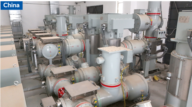
China | Hohhot Airport Substation Project
