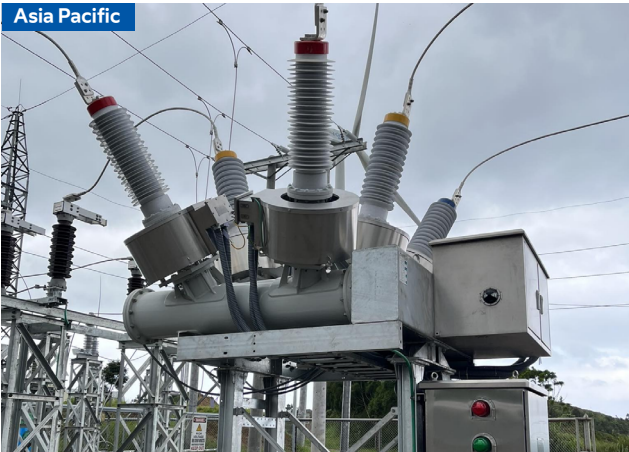
Philippines | 69kV Dead Tank Circuit Breaker Project
