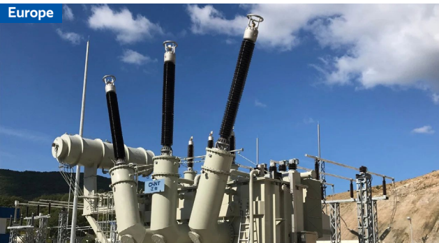
Montenegro | CGES 400kV Power Transformer Project
