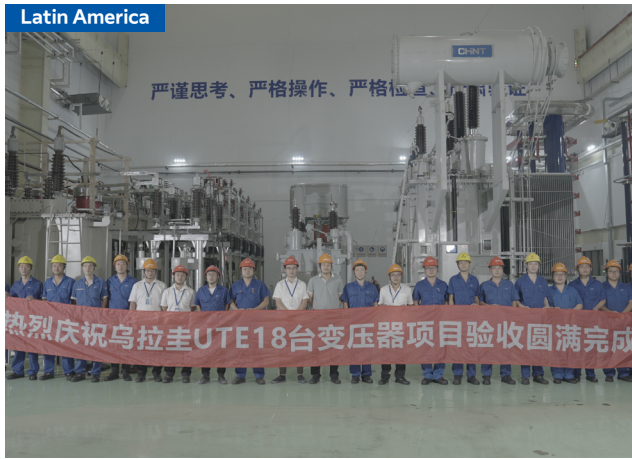
Uruguay | UTE 170kV Power Transformer Project
