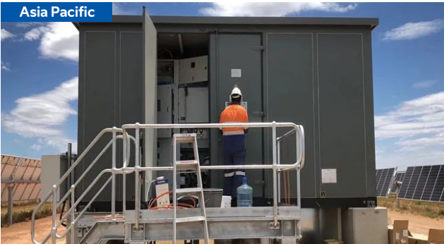
Australia | GreenGold 1074 Copper Coast Solar Farm
