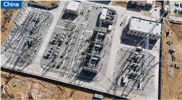
China | Inner Mongolia Power 500kV Substation Project
