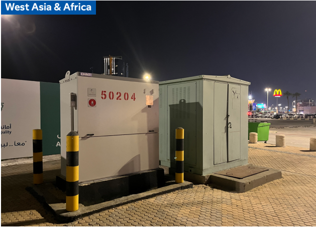
Saudi Arabia | SEC 17.5kV Smart RMU Project
