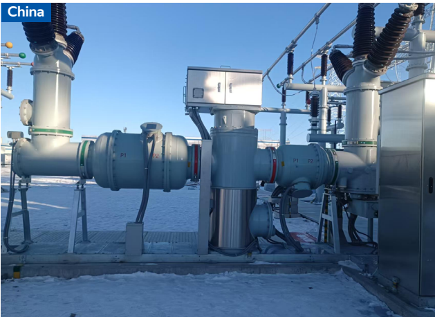
China | 550kV Yongquan substation 145kV GIS
