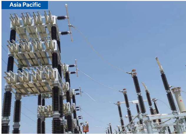
Afghanistan | Afghan National Grid Power System Upgrade Project
