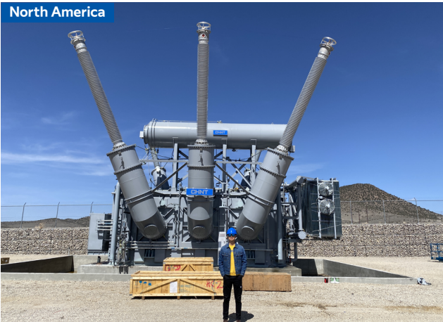
USA | 525kV 525MVA Autotransformer Project
