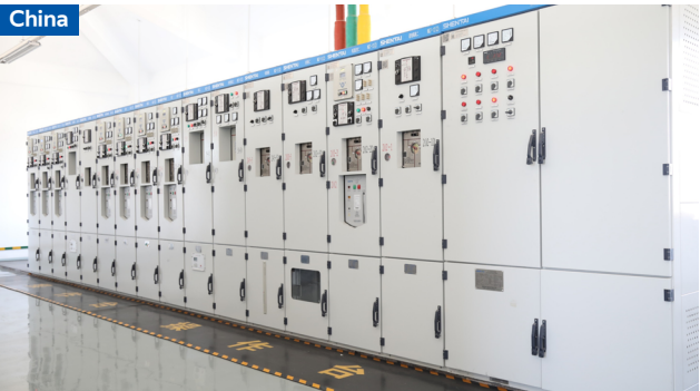
China | Beijing-Zhangjiakou High-Speed Railway 10 kV Power Distribution Substation Project
