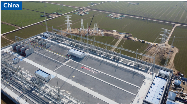
China | State Grid Xianxing 500kV Substation Project
