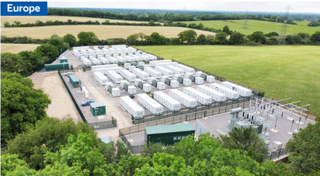
UK | Huaneng 99.8MW/98MWh Minety BESS Project
