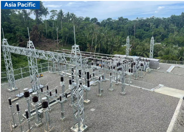
Philippines | National Power Corporation Mogpog Substation
