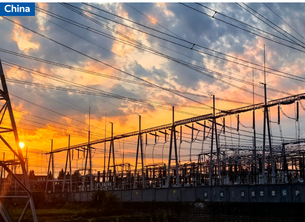
China | State Grid Nanchong 500kV Substation Project
