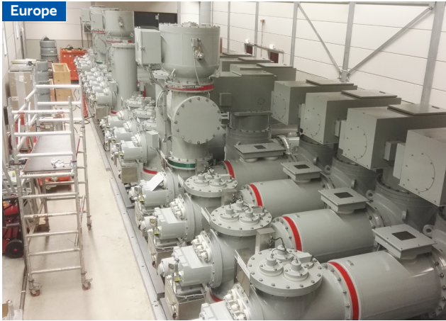
Netherlands | Alliander Amstelveen 72.5kV GIS Project
