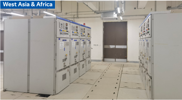
Egypt | 10th of Ramadan City Rail Transit Power Distribution Project
