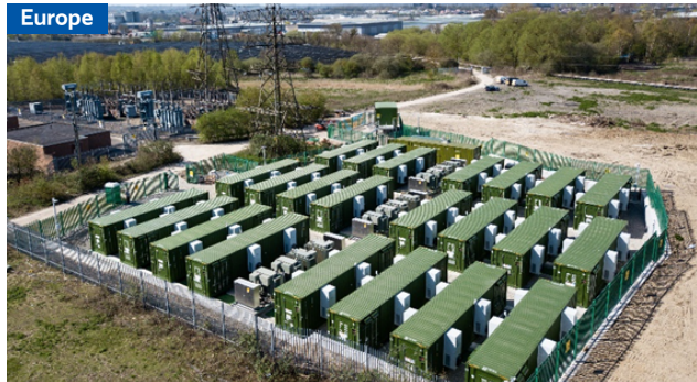
UK | BYD 159MW BESS Project
