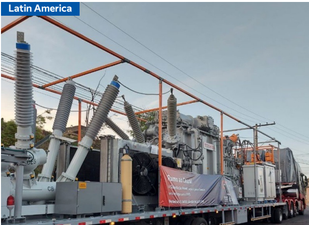
Brazil | CEMIG 145kV HGIS Mobile Substation Project
