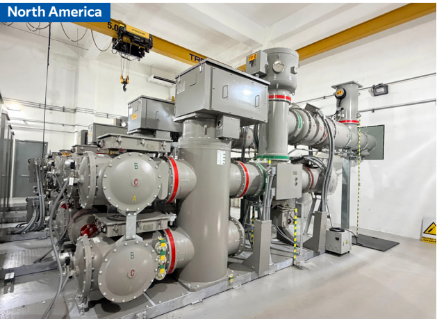
Mexico | SE CENTRO BANCO 1 Project 145kV GIS
