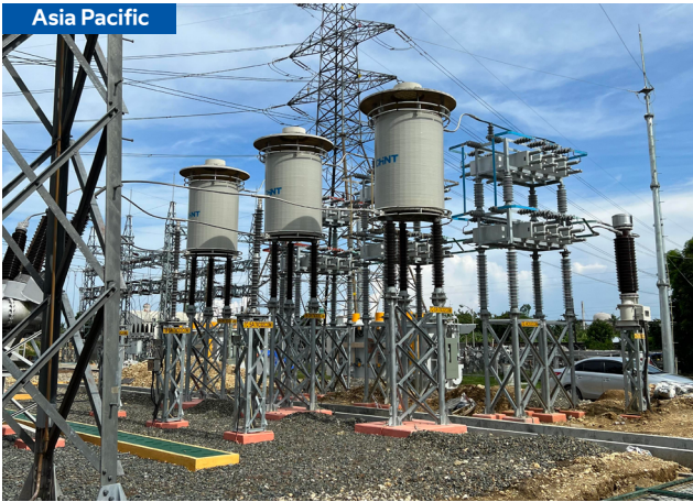
Philippines | Visayas Voltage Improvement Project
