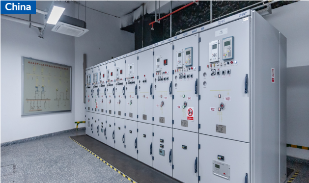
China | Hangzhou Metro Huanglong Substation Project
